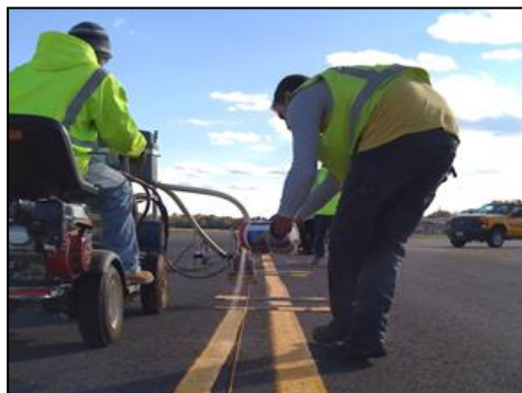
Right: A crew paints fresh lines on one of the airfield movement areas.
