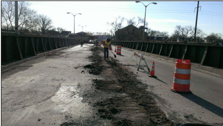
Left and Below: Lincoln Avenue Bridge (140.9) milling and resurfacing of deck complete rehabilitation.
