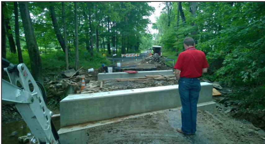
Left: Chris Markley, General Supervisor of the Highway Division's Roads Unit, examines the progress of the Van Dyke Bridge (234.1) reconstruction project.
