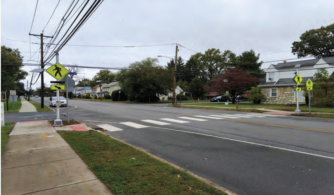
Pictured above: New audible Rectangular Rapid Flashing Beacon (RRFB) on Kuser Road in Hamilton Township installed by Orchard Holdings, LLC
