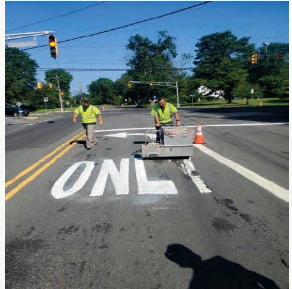
Pictured above: Lane directional marking restoration is performed at the intersection of Pennington-Lawrenceville Road and Blackwell Road in Lawrence Township
