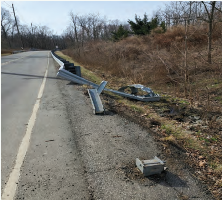
Pictured above: Basin Road in Lawrence Township hit and damaged by a truck accident
