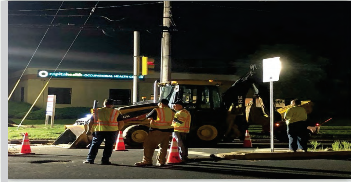
Pictured above: General Supervisor of Traffic Maintenance Mark Mattaliano along with Supervisor Traffic Maintenance William Heil assess conduit installation at the intersection of Quakerbridge Road and Village Road in Hamilton Township
