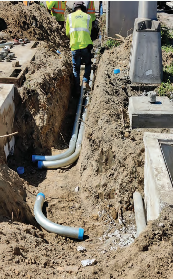
Pictured above: Electrical contractors laying rigid metallic conduit for new traffic signal at the intersection of Princeton Avenue and Mulberry Street in Lawrence Township
