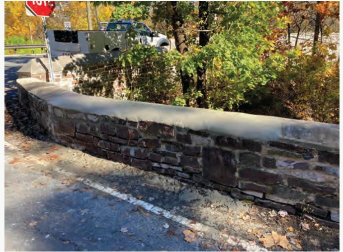
Pictured above: Replaced missing stone from parapet wall on Quaker Road, Bridge No. 330.2 in Princeton
