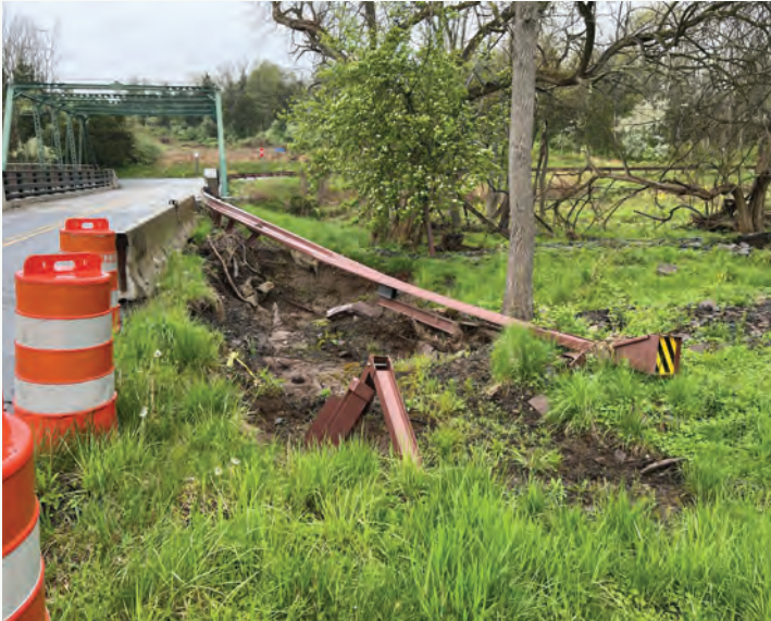
Pictured above: Valley Road in Hopewell Township washed out by Hurricane IDA in September 2021
