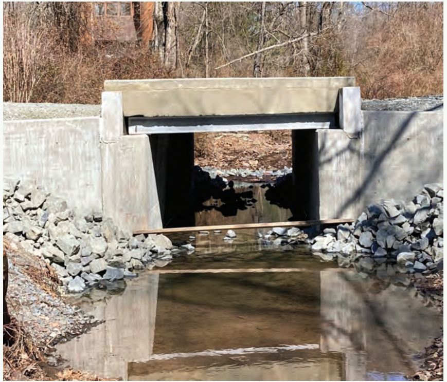
Pictured above: Completed in-house construction project on Bayberry Road in Hopewell Township
