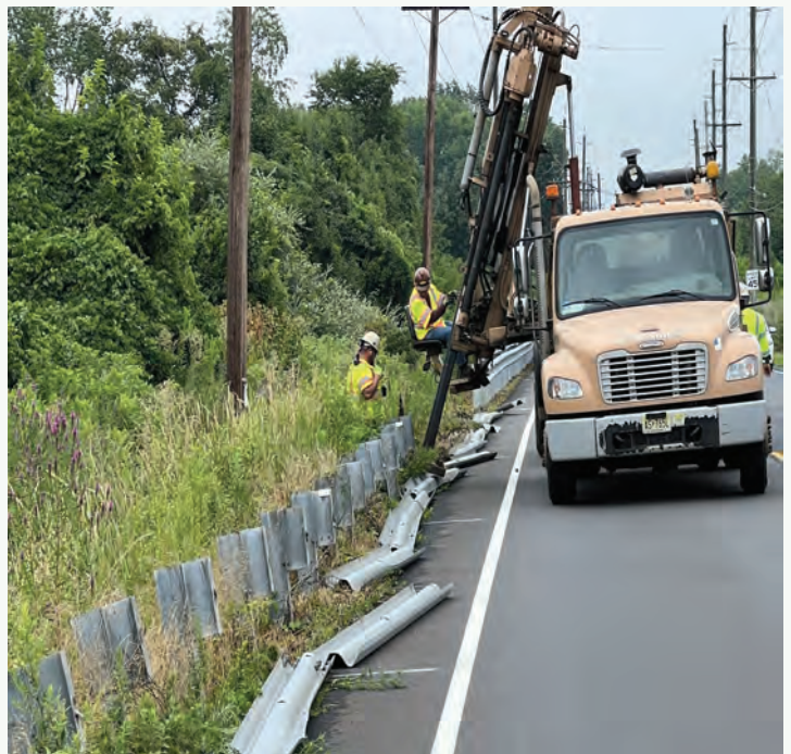
Pictured above: Guiderail on Clarksville Road in West Windsor Township under construction in August 2022
