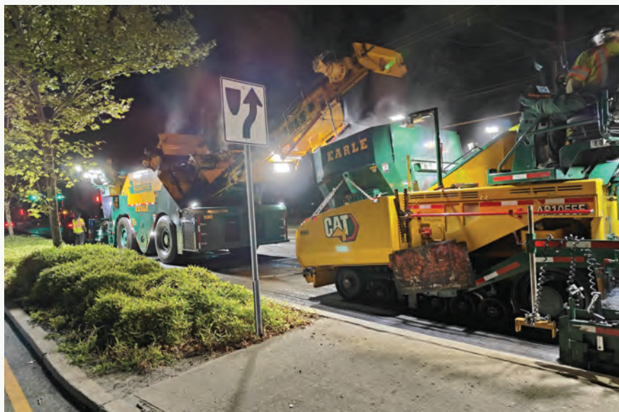
Pictured above: Earle Asphalt Company completing paving using transfer truck and paver on Whitehorse-Mercerville Road in Hamilton Township
