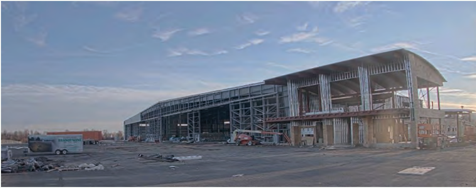
January 2022 – Roof is completed, outside walls are being installed and concrete working is ongoing
