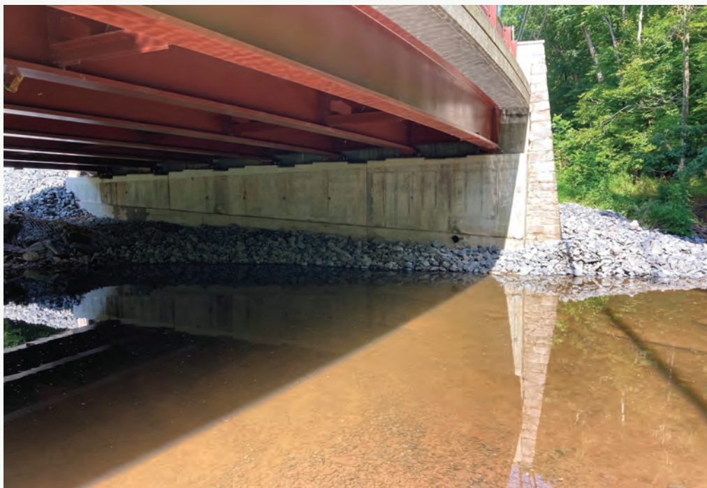
Pictured below: Installation of core stone on Bear Tavern Road, Bridge No. 214.2 in Hopewell Township
