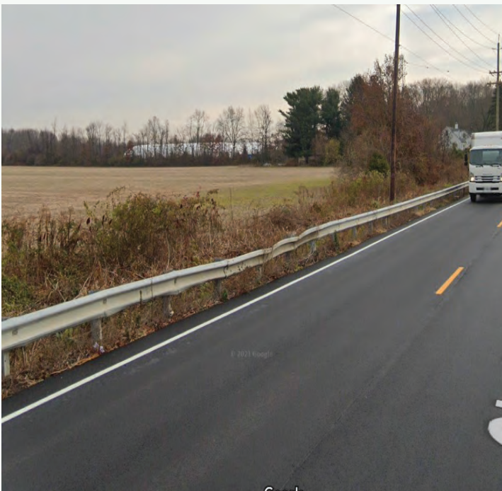
Pictured above: Guiderail on Clarksville Road in West Windsor Township in poor condition
