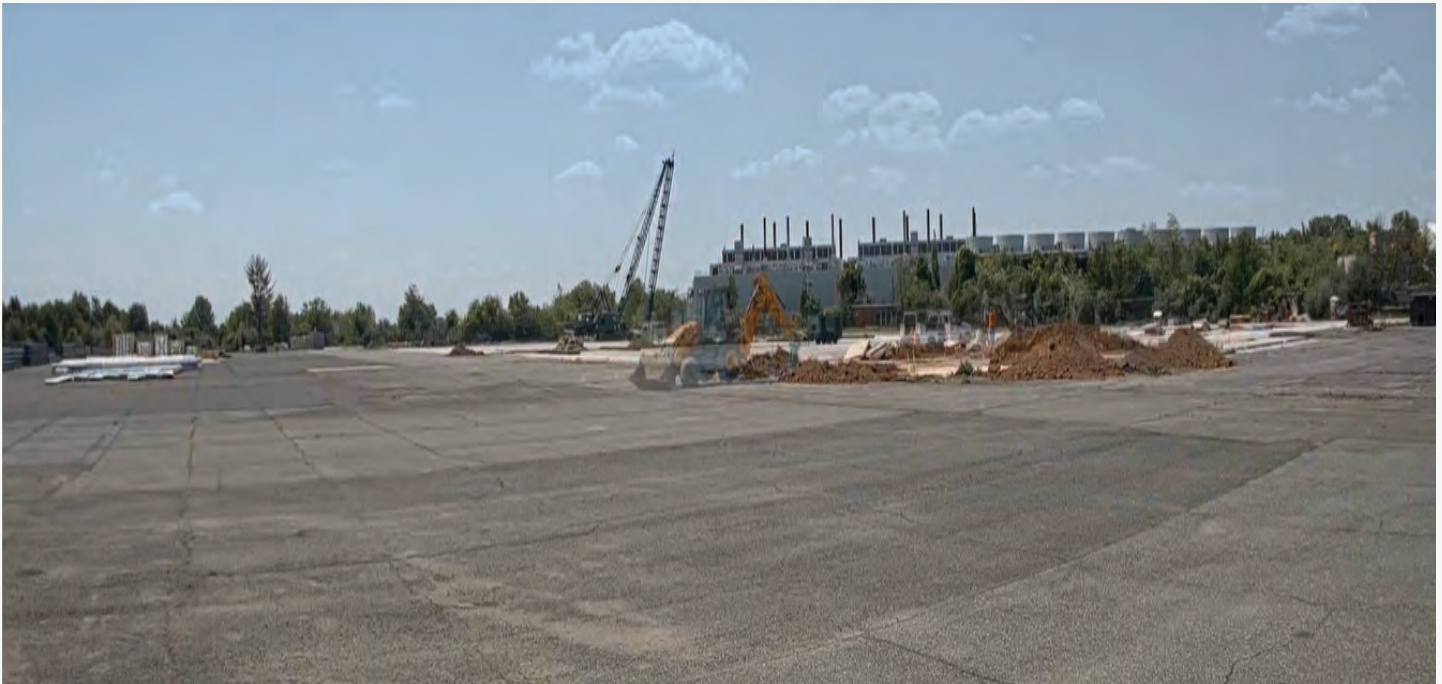
Pictured above: Old Navy hangar site after demolition and new hangar construction commencing
