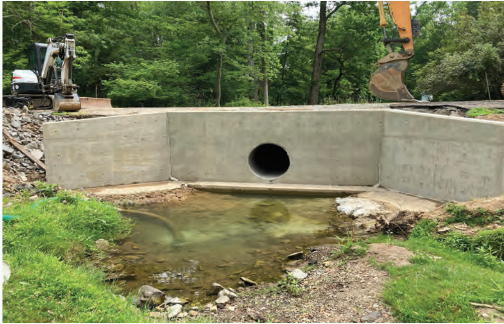
Pictured above: Replacement of culvert on Poor Farm Road, Bridge No. 213.9 in Hopewell Township; completed in-house
