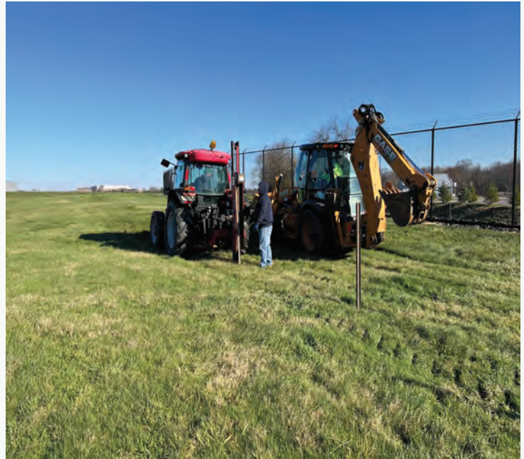
Pictured right: Installation of snow fence/poles. Prior to the onset of winter, snow fence is installed on areas that have the potential of snow to blow back on the roadway surface causing hazardous driving conditions.
