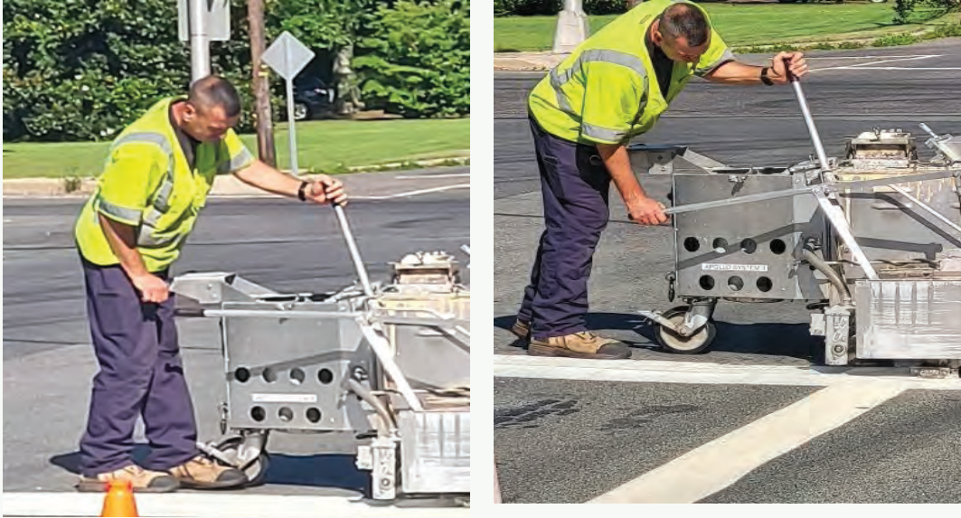
Pictured above: Traffic Maintenance Worker, Mike Gilleo uses caution while applying thermoplastic material onto pavement surfaces
