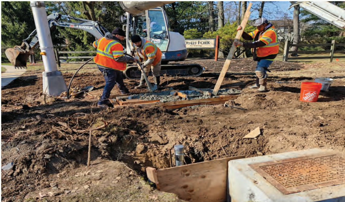
Pictured above: New Modified PMC Foundation for traffic cabinet being installed at Bear Tavern Road and Scenic Drive in Ewing Township by Orchard Holdings, LLC
