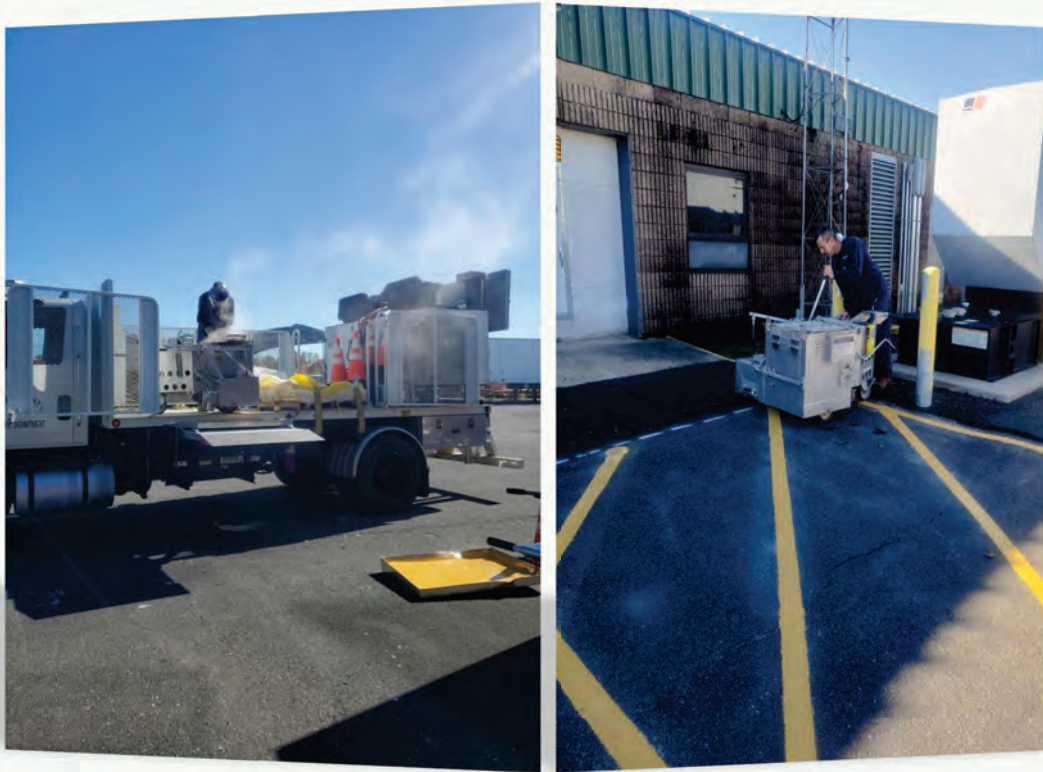
Pictured right: Yellow thermoplastic is heated and applied at the MCDOT complex for safety improvements along the buildings and grounds
