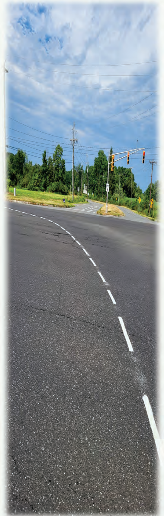
Pictured above: White thermoplastic lane divider markings successfully installed on Scotch Road per Capital Health Hospital's approved request
