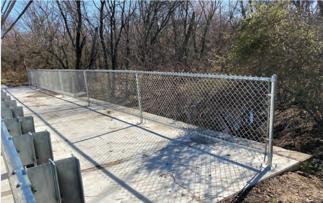
Pictured above: Installation of new poles and chain link fence on Edinburg Road, Bridge No. 641.7 in Hamilton Township
