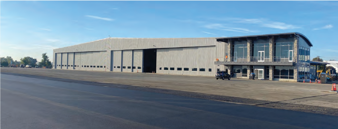
Pictured above: October 2022 – Completed construction of the new 80,000 square foot FlightServ hangar
