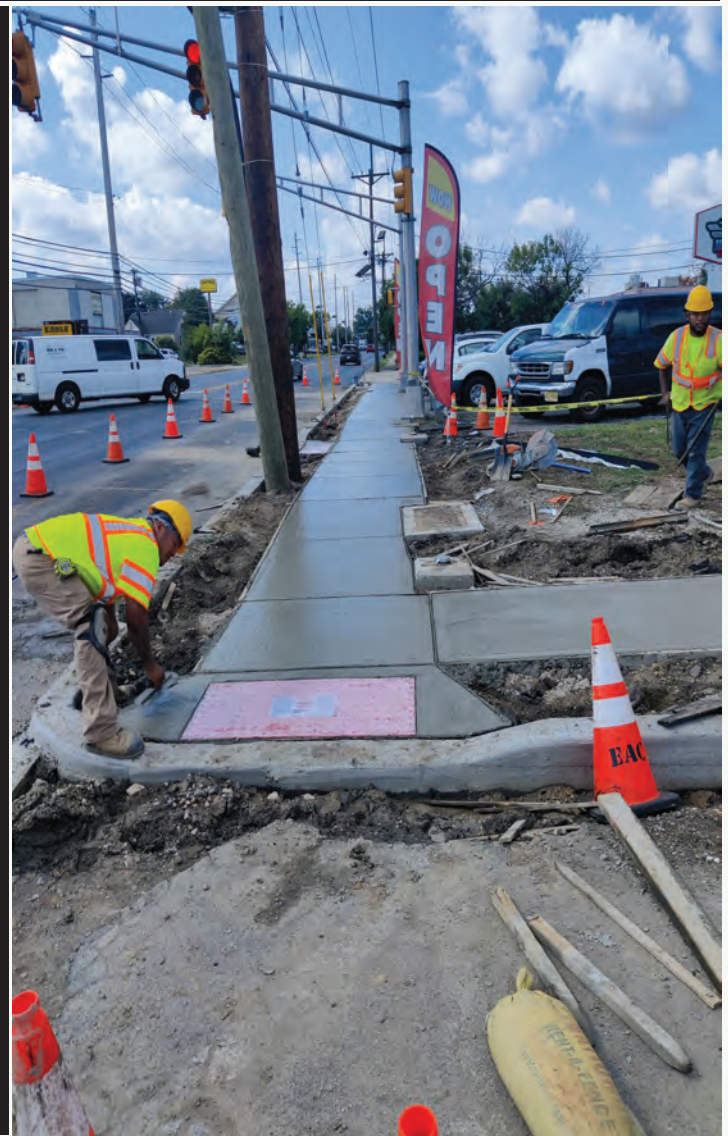
Pictured above: Concrete contractors laying new sidewalk at Princeton Avenue and Trenton Farmers Market Driveway in Lawrence Township
