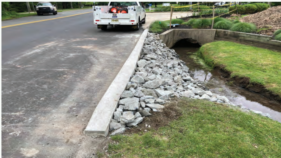
Pictured below: New concrete curb, along with installation of core stone at 1100 Franklin Corner Road in Hopewell Township
