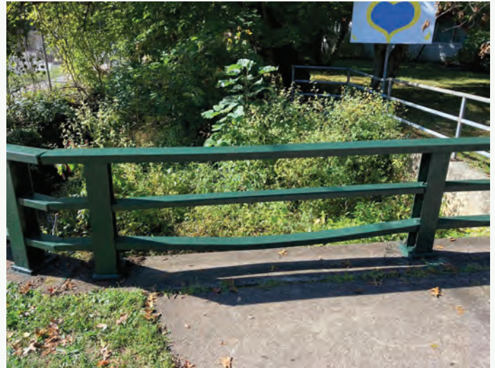
Pictured above: Replacement of angle iron on Fairfield Avenue, Bridge No. 541.6 in Hopewell Township
