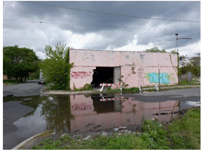
Drainage issue at W. Paul Street
