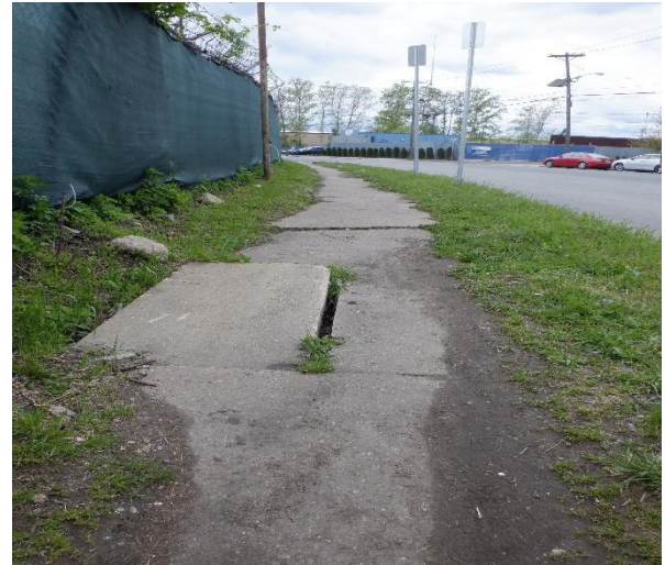
Deteriorating sidewalk along Calhoun Street
