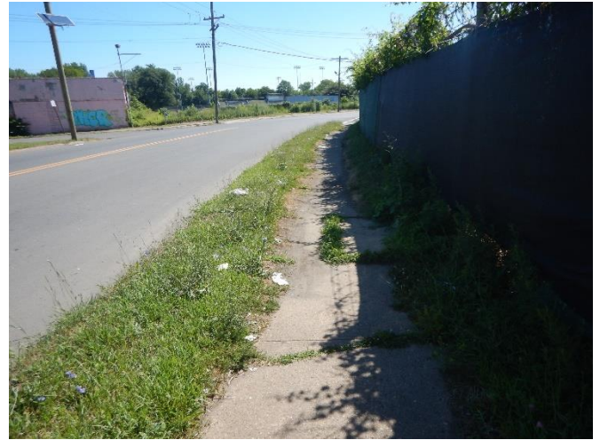
Deteriorating sidewalk along Calhoun Street
