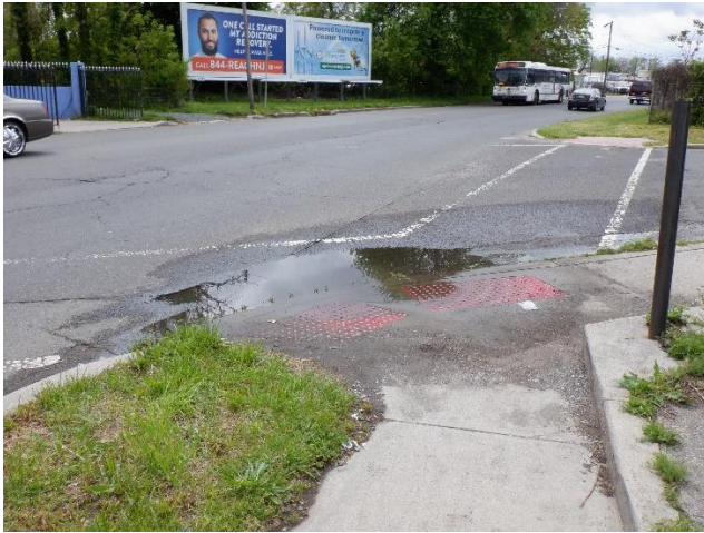
Ponding at ADA curb ramps
