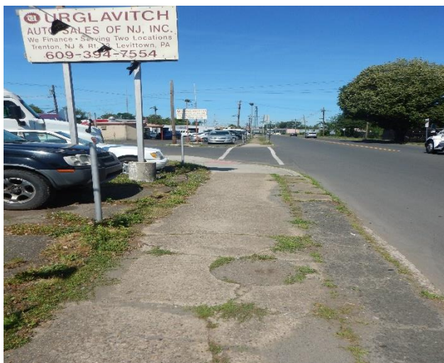
Deteriorating sidewalk along Calhoun Street
