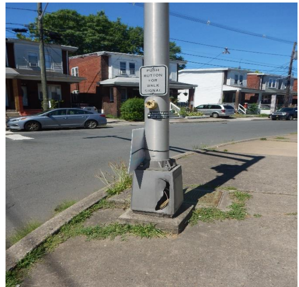
Damaged signal equipment at Calhoun Street and Southard Street intersection
