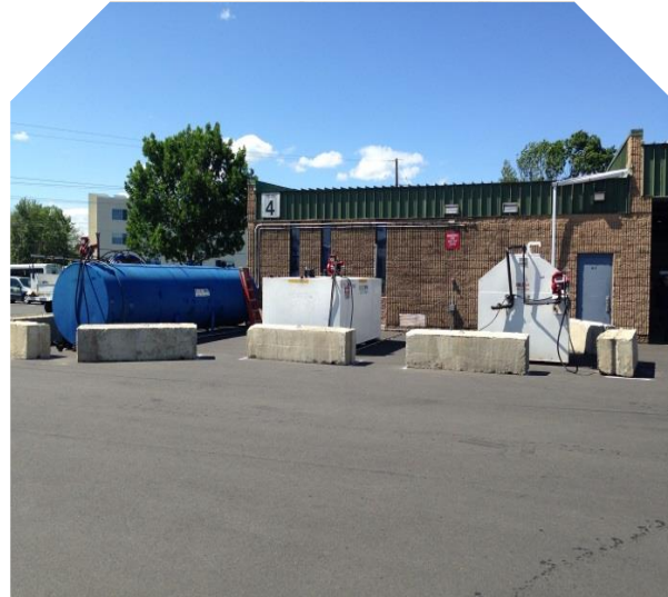
Temporary above ground fueling tanks Used in the interim
