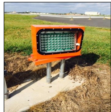
Trenton – Mercer Airport New runway indicator lights
