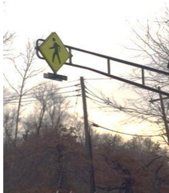
Rectangular Rapid Flashing Beacon
