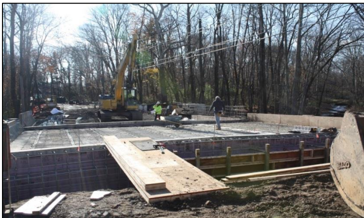
Carter Road (Bridge No. 543.7) Contractor Marbro, Inc. forming back wall of structure
