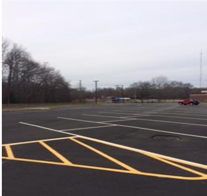
Interdepartmental Assistance Project Dempster Center Fire School Parking Lot Completed milling, resurfacing and striping
