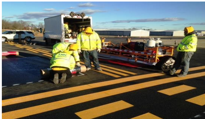
Installation of Thermo-plastic Surface Painted Hold Position signs on a taxiway. Thermo-plastic is a much more visible and durable material than paint.
